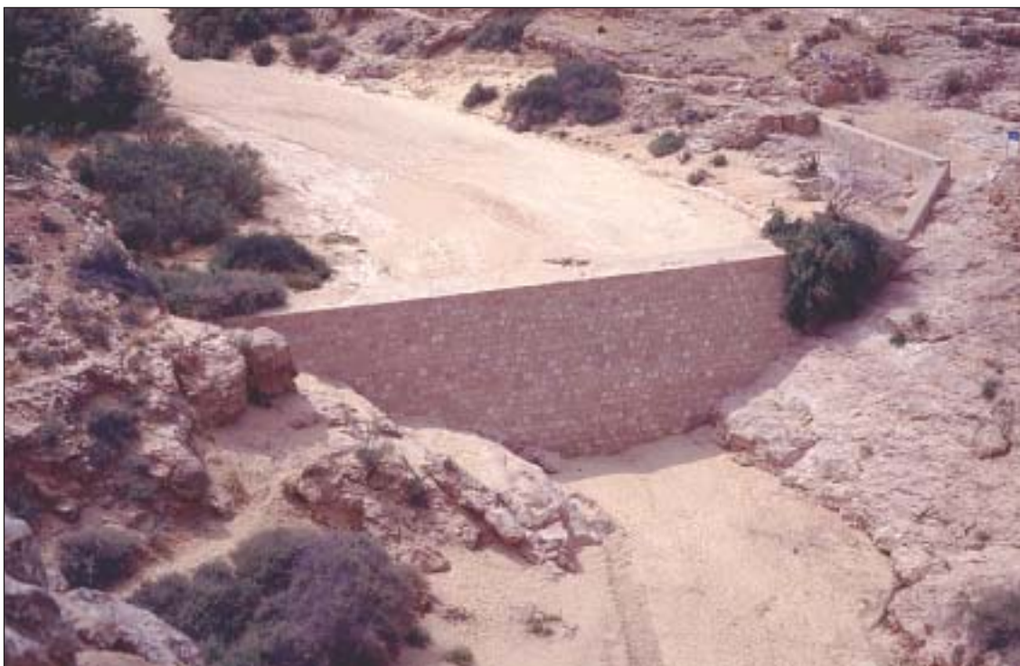
Reconstructed Nabatean dam across a wadi bed at Mamshit in the Negev. Such dams were part of a sophisticated irrigation system that enabled the Nabateans to practise agriculture in desert conditions.
