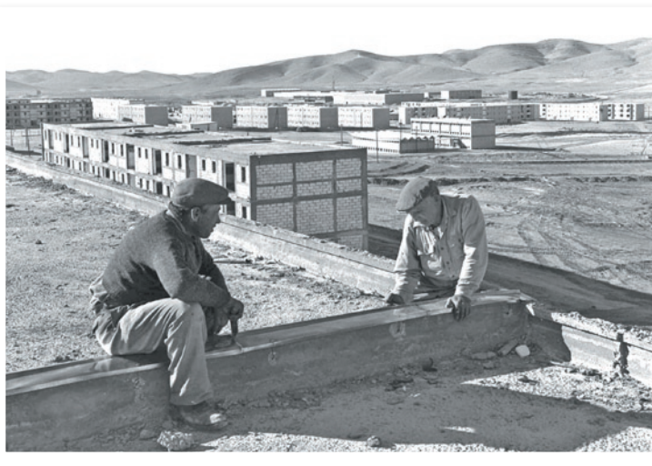
Houses under construction in Dimona. It was at this development town in the Negev that Israel built its nuclear facilities.
